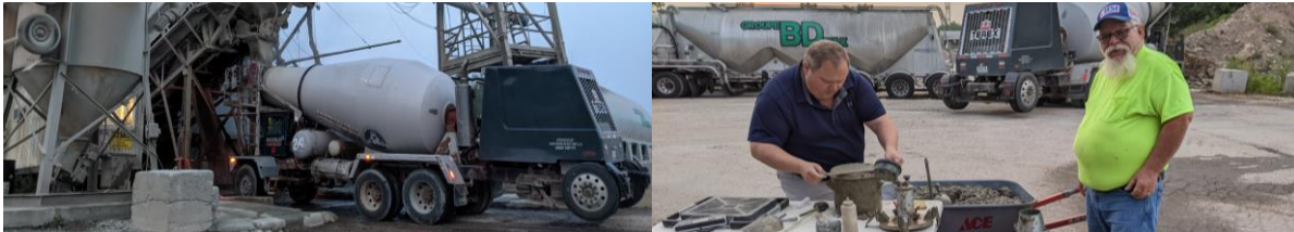
Figure 3: Batching and field testing at Riccelli-Northern Monday morning as the project commenced.
