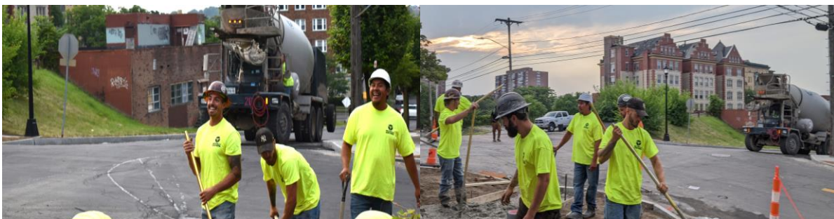
Figure 4: The Crew from McConnell Concrete at the corner of N McBride and E Willow Street.
